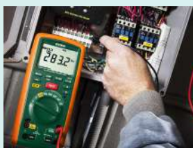
Voltage check on motor starter
