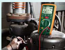
Insulation test on pump motor
